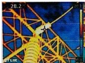
Gambar 2. Uji Thermovisi Clamp PMS Buss II Arah Busbar
