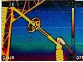
Gambar 3. Uji Thermovisi Kontak PMS Bus II
