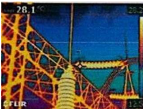
Gambar 6 Uji Thermovisi Terminal Post Isolator II Arah Busbar .
